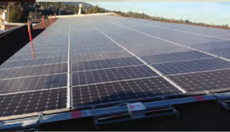
Solar panels newly installed on top of worship center
